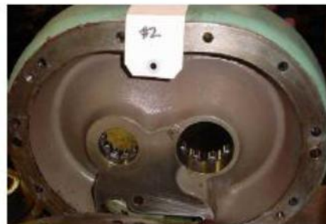
Inlet Rotor Average Varnish: 9.8 Sludge: 9.5
